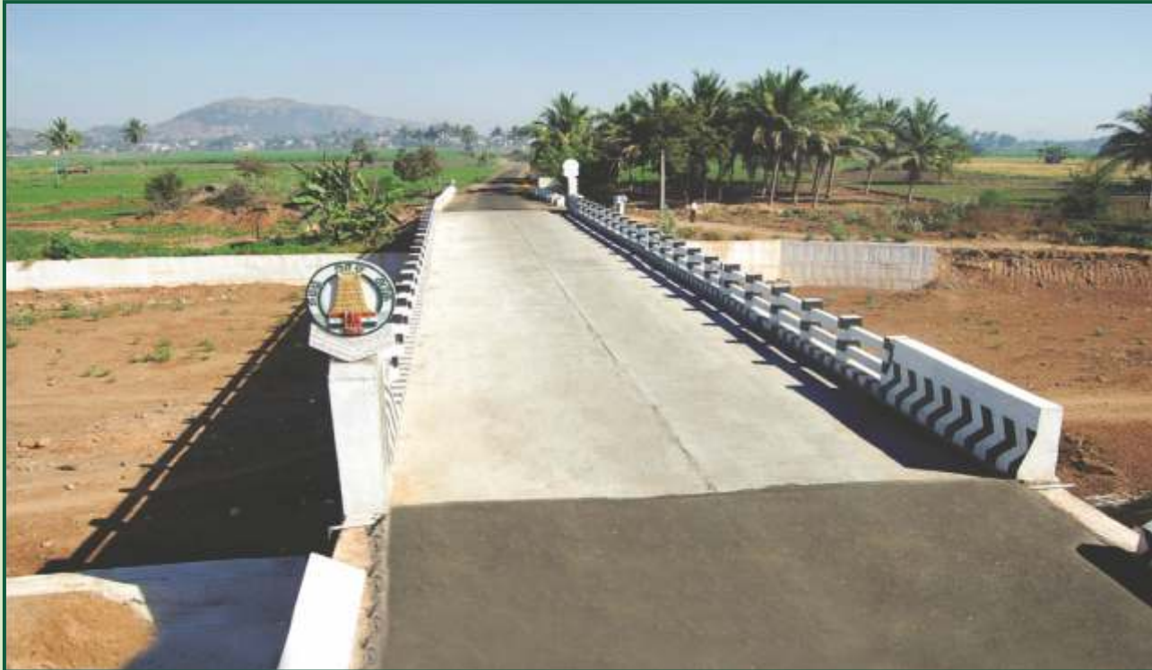
Construction of Bridge under Scheme Component of Pooled Assigned Revenue Villuppuram District
